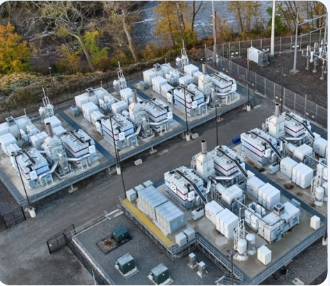
14 MW - 2023 Connecticut: Utility
