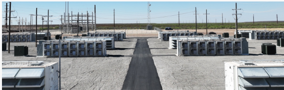
Bravo (2022) Deployed utility-scale compute at fraction of industry cost and time
