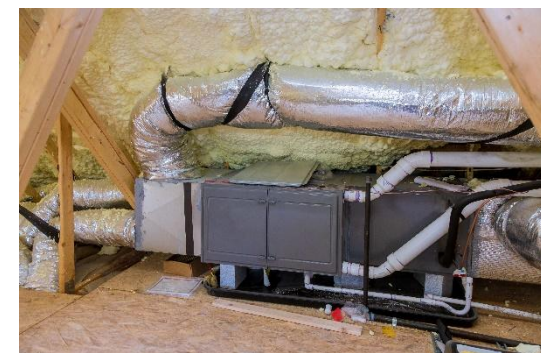
HVAC/R / Climate Comfort
