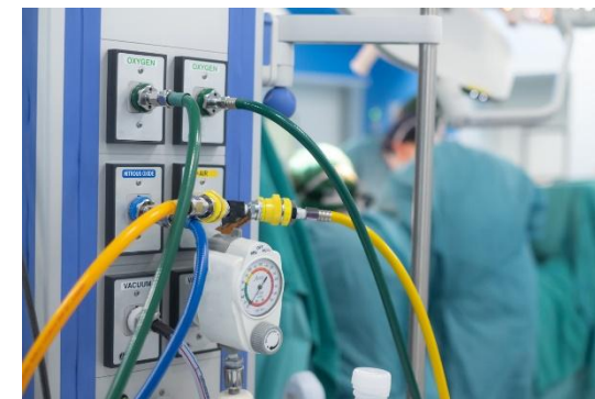
Medical Gas Distribution
