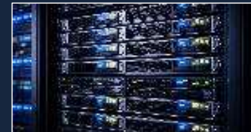
General Purpose Servers
