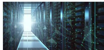
Data Center / Networking ("DC/NW")
